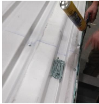
Figure 21: Base Angle Void
