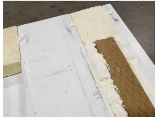
Figure 52: Structural lumber installed in flute above wall sealed with Sika-Flex and spray foam and fastened with deck screws.
