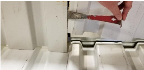
Figure 14: Trim Pry Bar used to help start inserting the tenon side into the channel side of the previous panel
