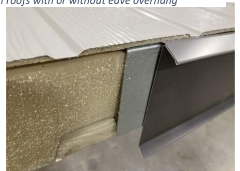
Figure 58: Kerf cut in the roof eave to accommodate fascia trim and eavestrough supports
