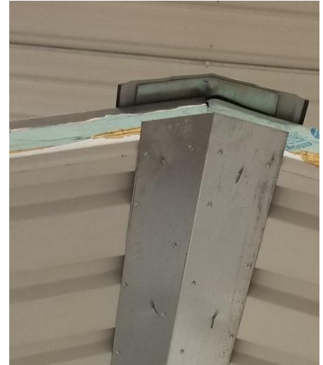
Figure 56: Ridge cap, top and bottom ridge support angles with roof panels sandwiched between
